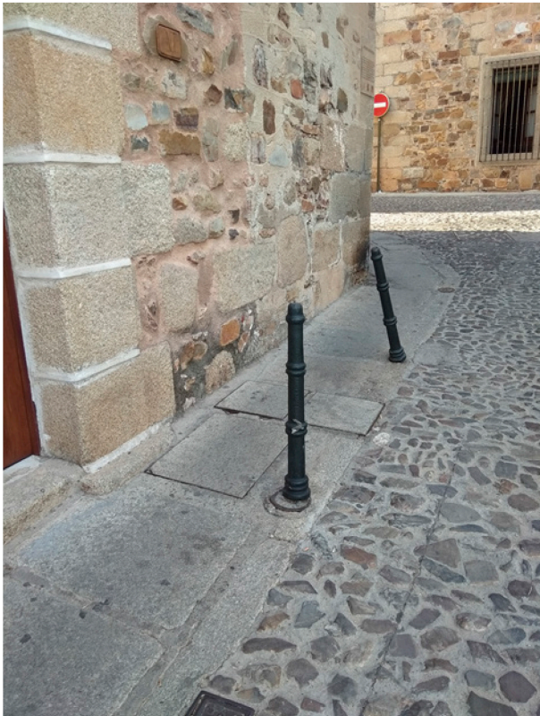
Fig. 4. Typical pavement .Stretch three of the proposal itinerary at Puerta de Mérida. (Source: Own, 2020).
