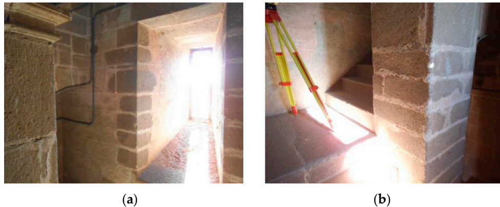
Figure 10. Walls built with granite ashlars (a,b). Interior of Santa María Church, Guareña (Spain).
