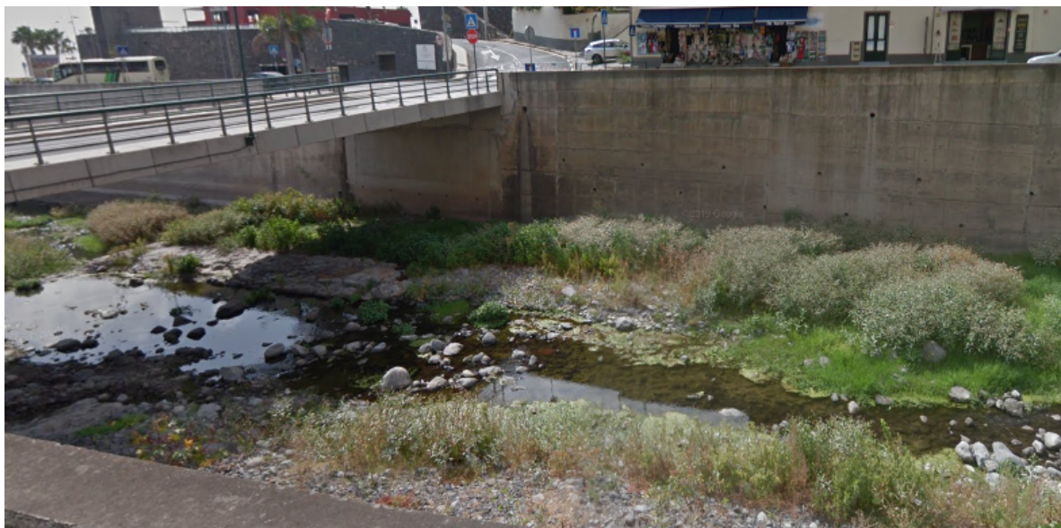
Figure 2. State of conservation of Ribeira Brava main watercourse river mouth.
