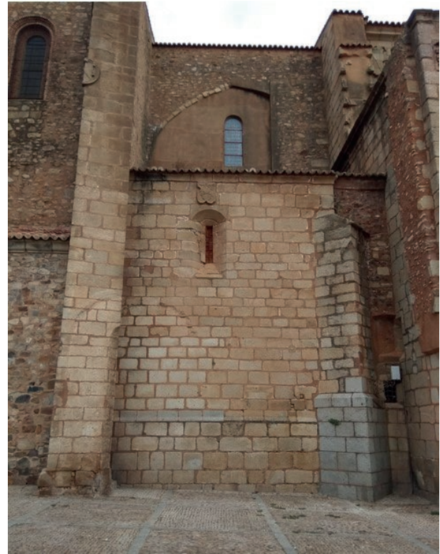
Fig. 16. Detail of the south façade, without the chapel and the warehouse that disappeared in 1980. 2022. Photo by the author.
